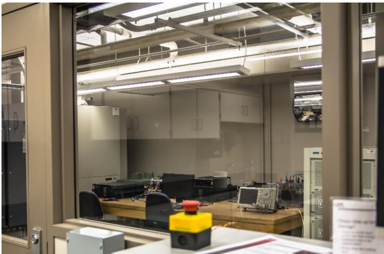
The High Power Area (Hybrid Microgrid Testbed)
